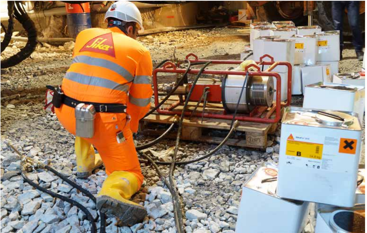
Application of SikaFix®-210 using a two-component pump and compressed air from the mine.
