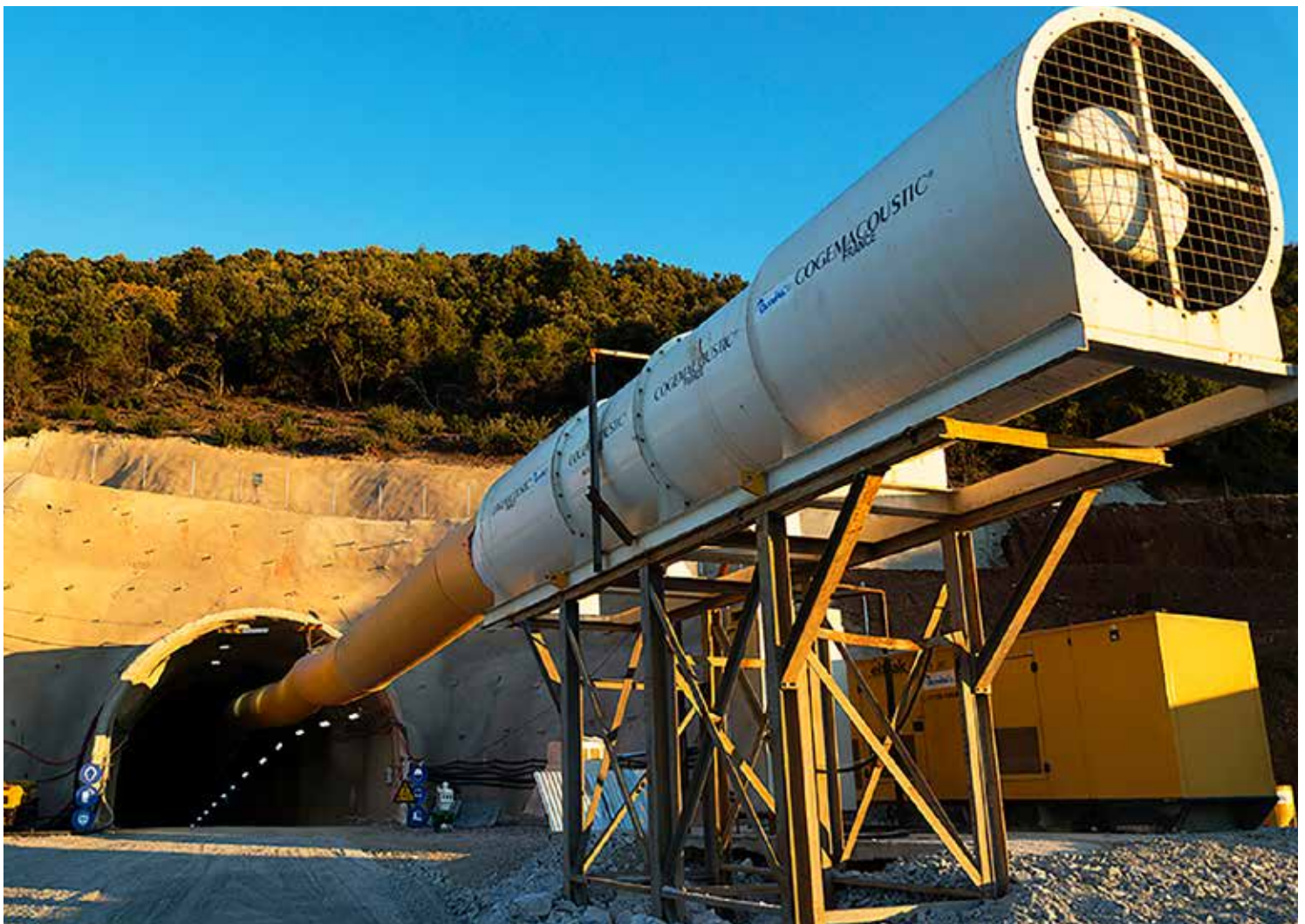
The stratoni-olympias decline portal and ventilation equipment.
