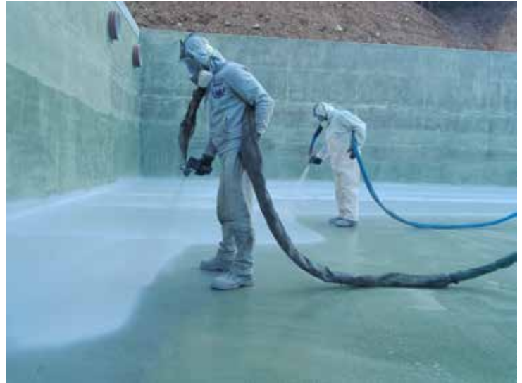
The two-component, liquid, hot-spray, polyurea based membrane Sikalastic®-843 GP is applied at the surface reservoir of the Kokkinolaka mine.
