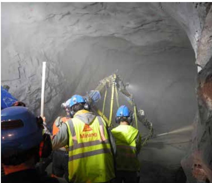
Sika® Sigunit® shotcrete accelerators and concrete admixtures are used for all of the Kassandra underground operations and allow rapid mine cycle times for fast underground development.
