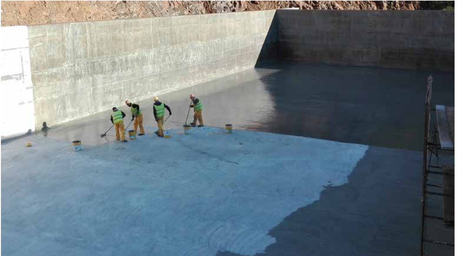
Application of the two-component Sikafloor®-161 epoxy primer followed by Sikafloor®-161 scratch coat.
